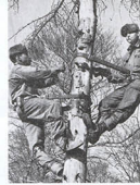
A pair of 3d AFA Bn wiremen setting the communication wiring that is so vital to artillery during a field problem.
